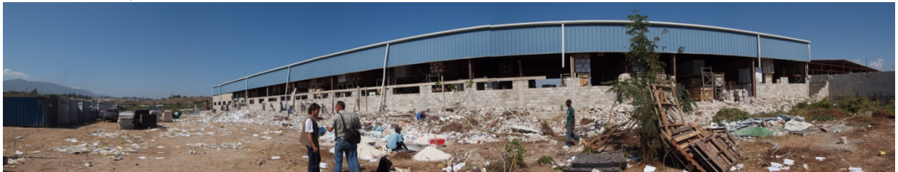
Figure 1 Collapsed wall in rear of PROMESS warehouse, February 2, 2010
